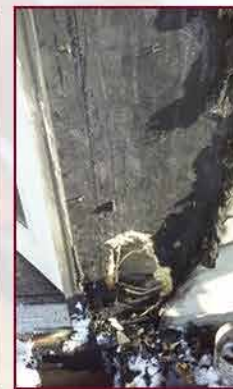
Roof Vent Fire
