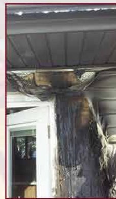
Gutter & Siding Fire
